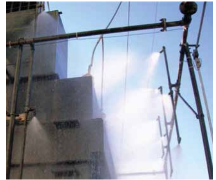
Deluge water spray system
